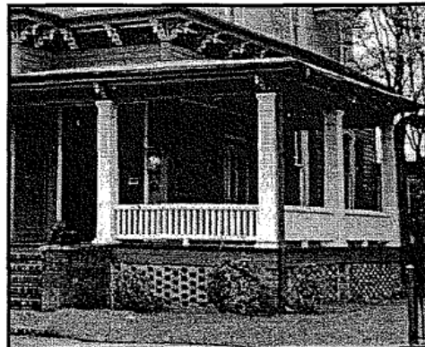
The brick pier foundation of the Mansard Roof House has been infilled with lattice-patterned brick. The wall retains the original wood siding and decorative details.
