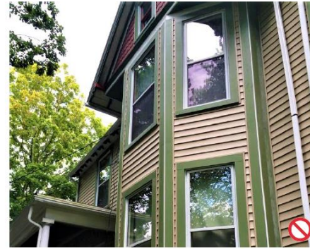
The corner stripping required for the vinyl siding on this house negatively alters its character.
