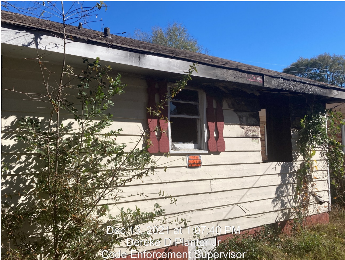
(flashing and trim/fascia damaged and burnt; roof rafters and sheathing need repair)
